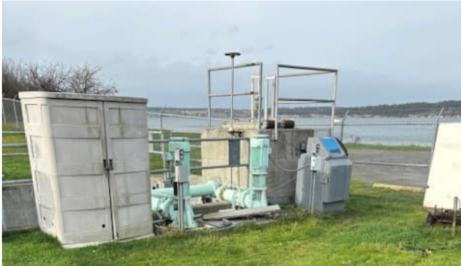
Figure 4-2. Existing WWTF Outfall Pump Station
