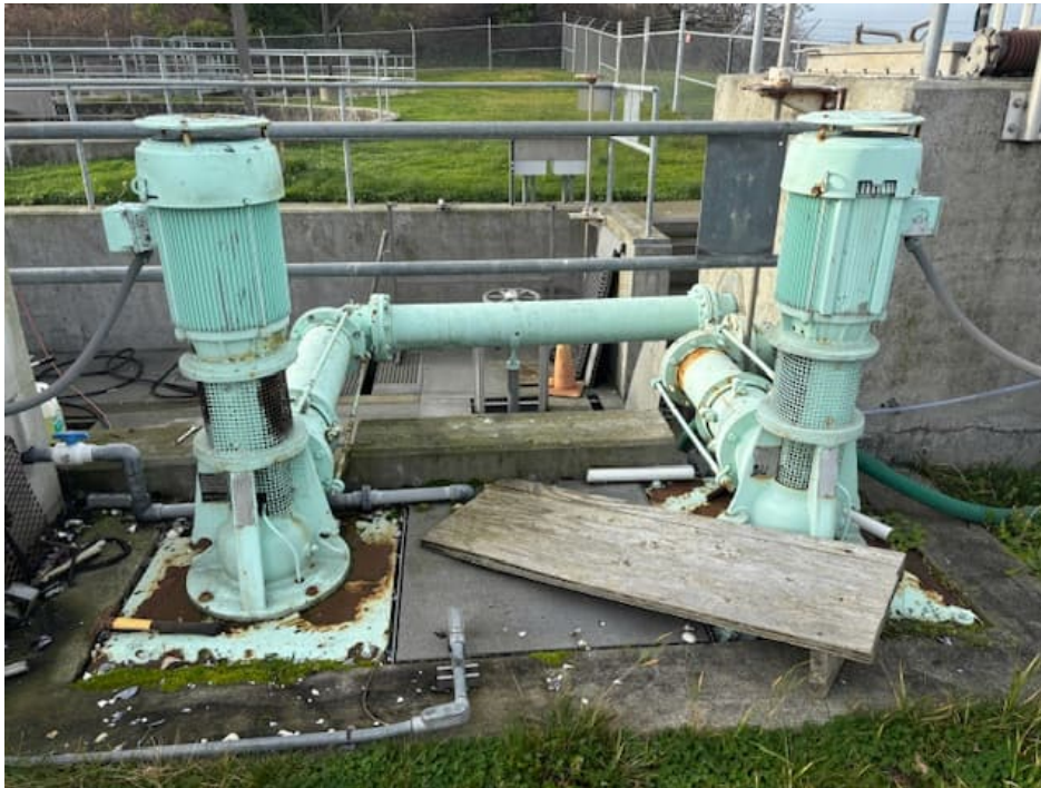
Figure 4-3. WWTP Outfall Pump Station with a Third Pump Bay between Two Existing Pumps
