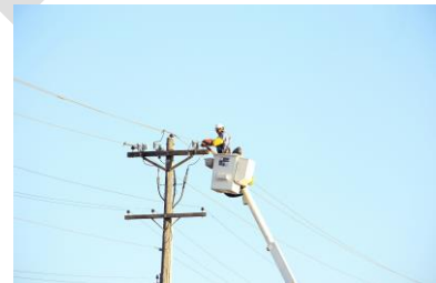
Electrician working with a utility pole (photo credit: American Public Power Association).
