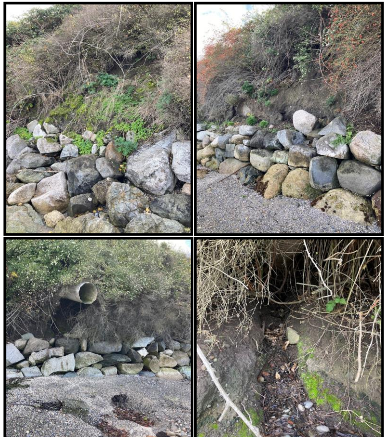
Figure 22. Site photos of eroded bluff above existing rock revetment (top) and the stormwater outlet associated with erosion above the rock revetment along NE 9 th Street (bottom).
