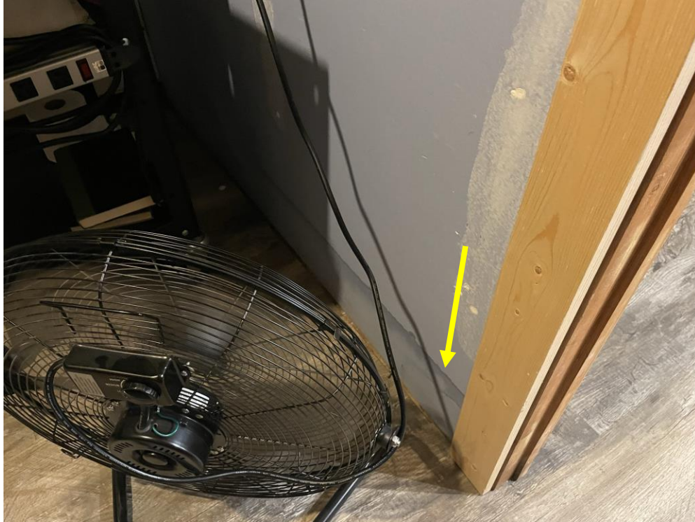
Figure 28. Flood level (see arrow) within one of the Front Street commercial buildings lower floors from the December 27, 2022, regionally historic high-water event (Photo Credit: Avery Maverick, 2023).
