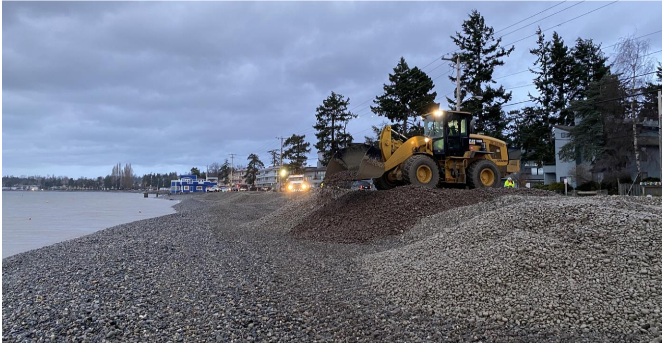
Figure 2. Example of large-scale beach nourishment project in Birch Bay, WA to mitigate coastal flooding and erosion. Larger than native sediment was utilized to dissipate wave energy and help to form a high berm for storm protection (Photo Credit: Jim Johannessen, 2020).
