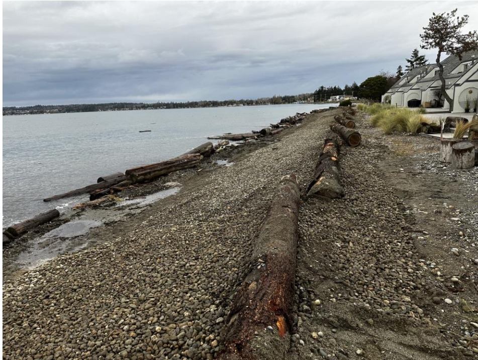
Figure 3. Example of large wood anchored on the beach to protect adjacent houses from coastal erosion (Photo Credit: Adam Tullis, 2024).
