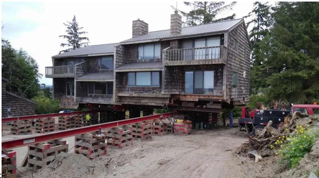
Figure 13. Example of structure relocation on Whidbey Island (Photo Credit: DB Davis LLC).
