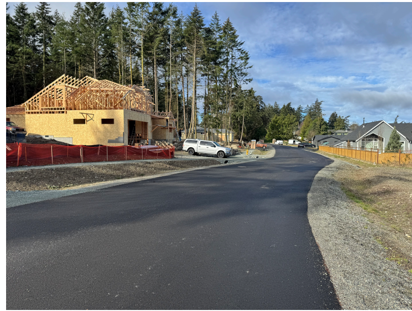
View to the West from street in front of project Lot 2 / 207 NW 3rd Street.
